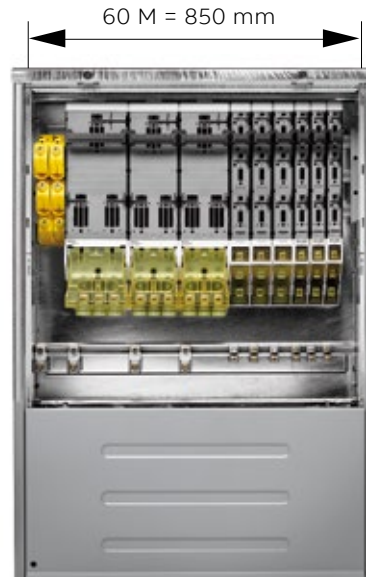
Module dimensioned busbar system in the cable distribution cabinet.
